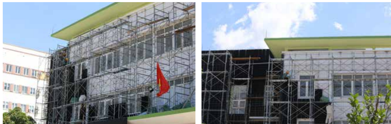
Figure 27: The steel support system and modules of the green wall were being installed Source: © Luong Thanh Trung/ GIZ
