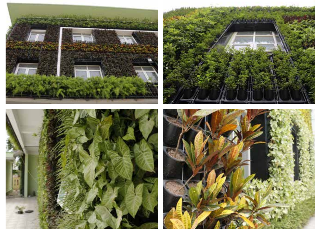
Figure 24: The green wall vegetation cover of the measure Source: © Luong Thanh Trung, Trinh Ngoc Quynh/ GIZ
